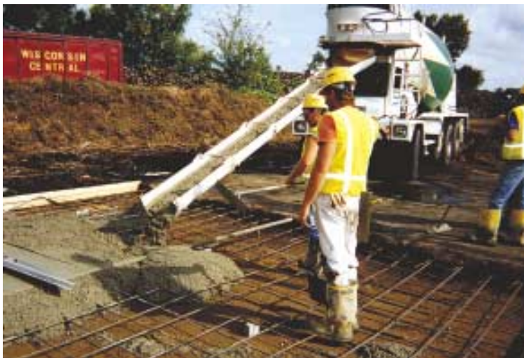
Fig. 1: Workers ready to place fresh structural-grade wood-ash concrete for a demonstration slab in Rothschild, Wis.
