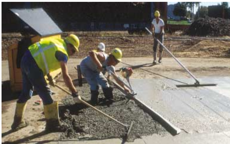
Fig. 2: Finishing the demonstration slab of structural-grade concrete incorporating wood ash, placed in 2001
